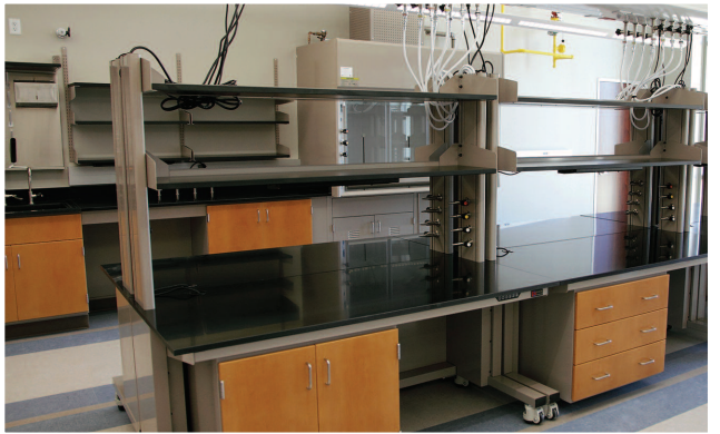
Overhead service enclosure with quick connect fittings
