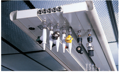
Overhead Service Manifolds
